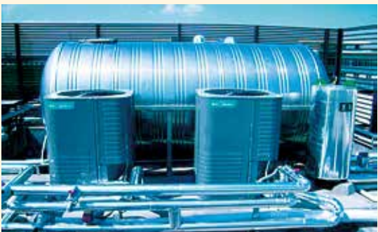
Project: Jiaxing Nanhu Technology Center Model: RSJ-380/S-820x2 RSJ-200/S-540Vx2 Water Yield: 30 Ton/day
