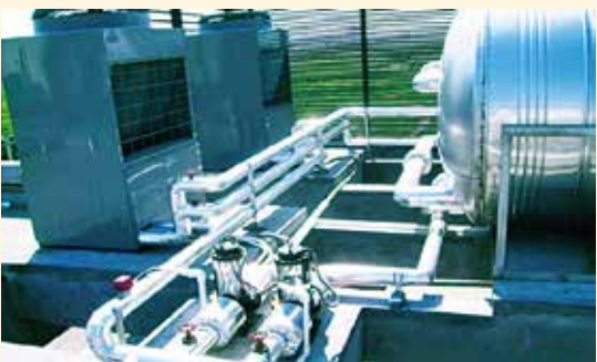
Project: FED International Corporation Model: RSJ-380/S-820x8 RSJ-200/S-540Vx2 Water Yield: 90 Ton/day
